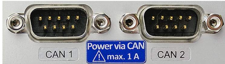
The DSUB-9 sockets are labeled.
